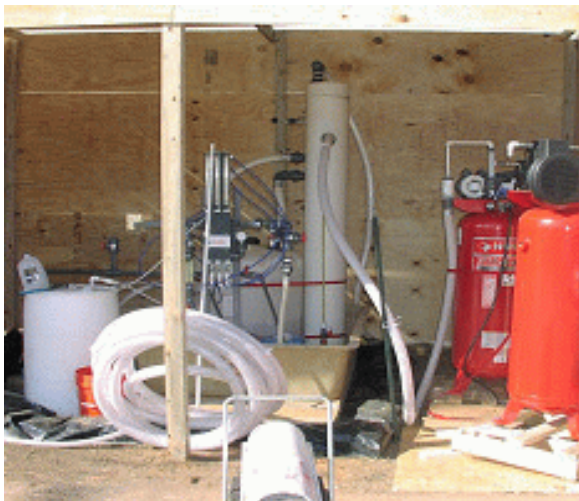
Figure 5.1-6a. Chlorine Dioxide Generation System at Beltsville, MD
